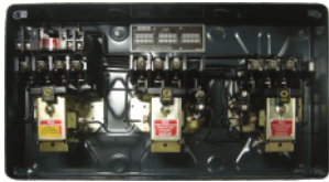
Interior View of MK1 SASD
