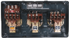
Interior View of MK2 SASD
